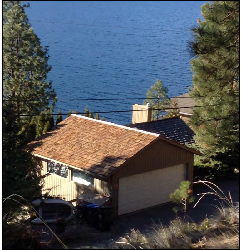
Figure 13. New shake roofing in the North Clifton neighbourhood. Mature pine trees adjacent will likely contribute additional combustible material to the roof, if allowed to accumulate.
